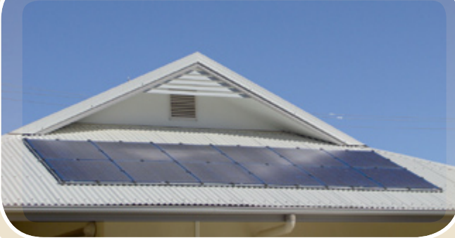
Photovoltaic (PV) cells help reduce your impact on the environment
